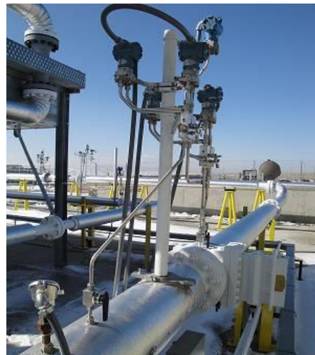
Figure 7 – 8" 0.564β Orifice Meter
